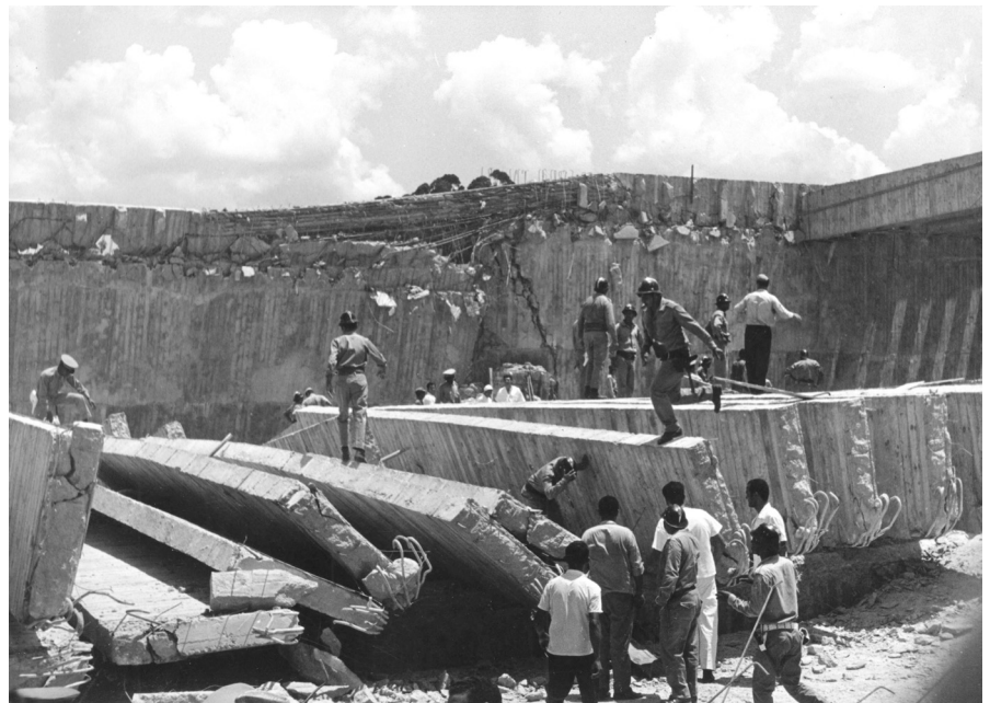
FIG. 8 Gameleira pavilion, Belo-Horizonte, construction collapse February 4, 1971.
